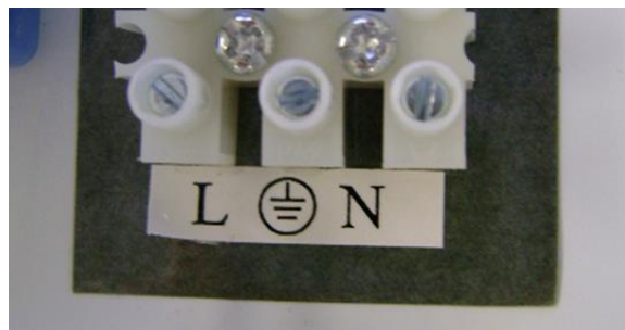
Terminal block marked with L, N, and earth symbol
