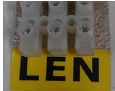
Terminal block marked with L, N and E indicating the "E" terminal is provided for the termination of the supply conductor but not connected to the luminaire e.g. class 2 product.
